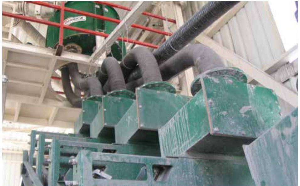
One of thirteen Derrick Stack Sizers successfully implemented at Esan Eczacibasi's lead and zinc operations at Balya, Turkey
