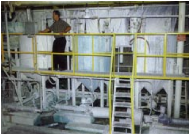
Process engineer M.J. Quellte monitors the coating kitchen control panel at Badger Paper's Peshtigo, Wis., mill. Three progressive cavity pumps (below) transfer each batch from the three-tank system to the paper machine, while a fourth (not shown) transfer solutions from mix tanks to the first coating tank.
