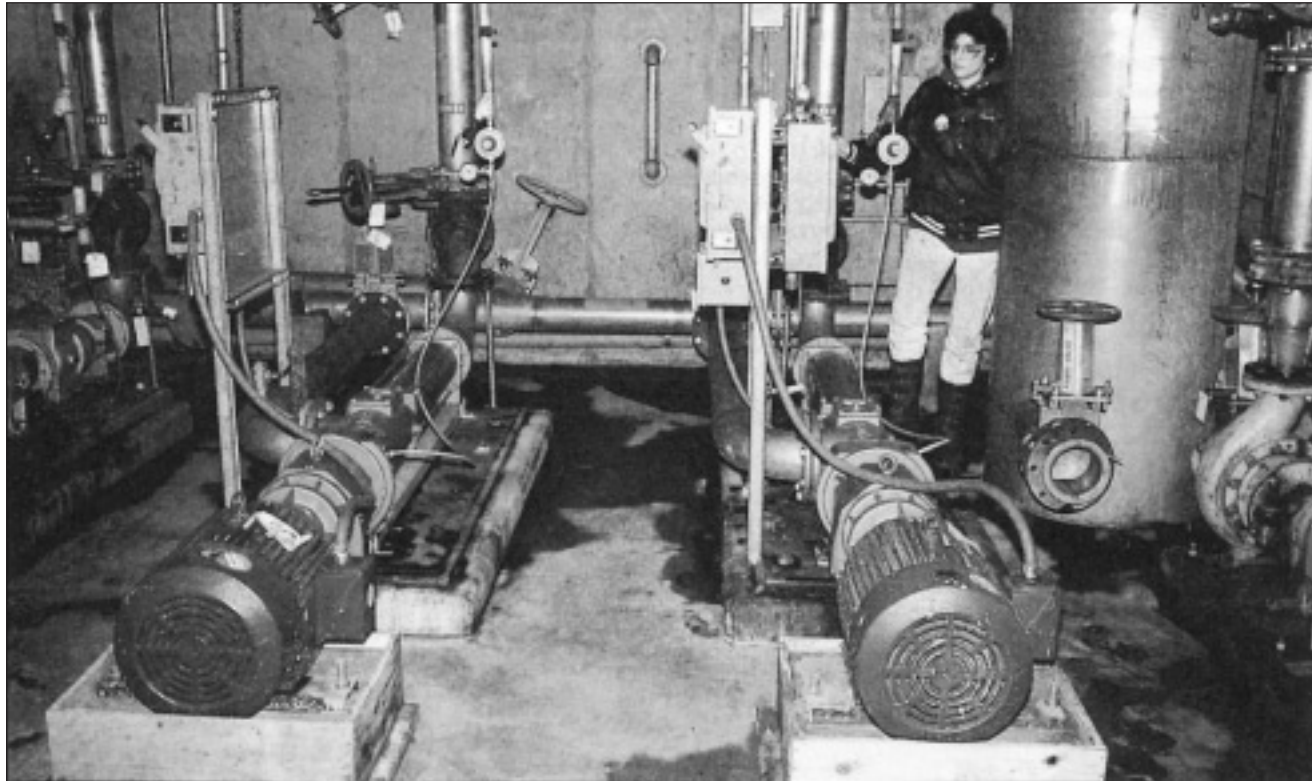
Two new progressive cavity pumps transfer sludge from final storage tanks to dewatering at Menominee Paper's wastewater treatment plant in Menominee, Mich.
